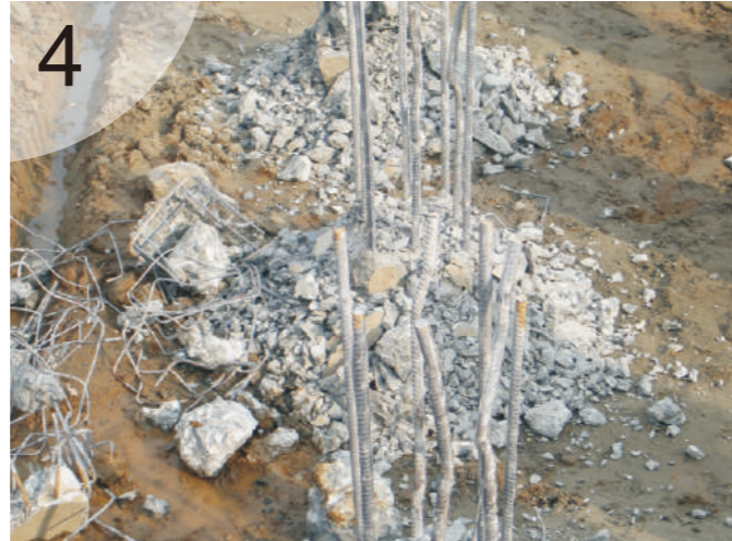
完整拔出 The final result is the perfect cleaning of the reinforced structure while the structure of the pile remains unchanged without creating cracks on the lower part which is still below ground.
