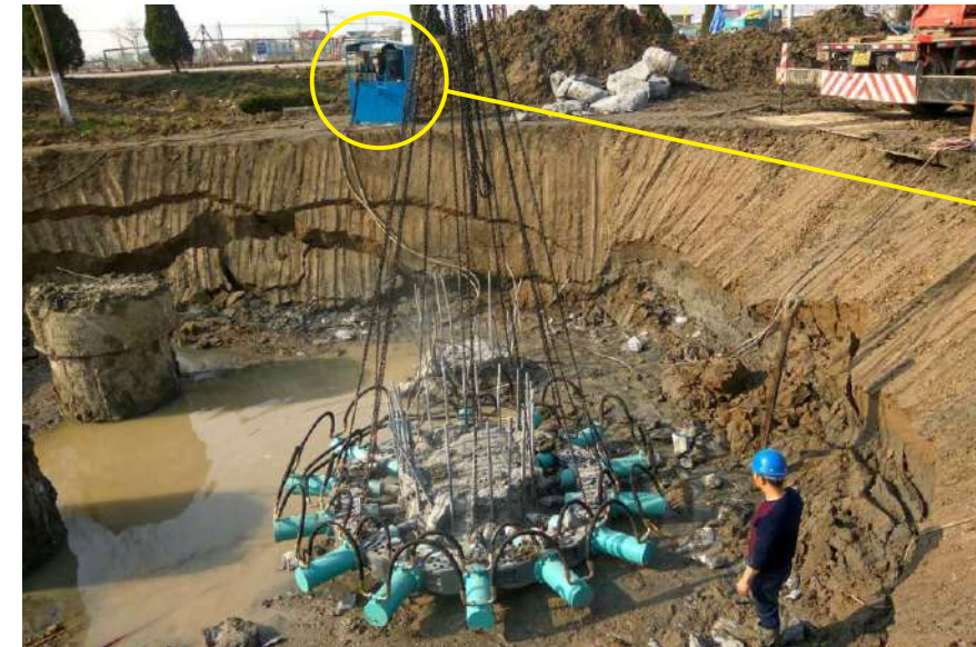
液压站 Hydraulic power station
